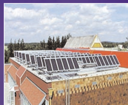
Swimming pool heating
