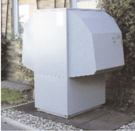
Air source heat pump (ASHP)
