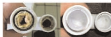
Descal for urinal pipes
