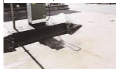
Heavy oil cleaning – after DeepClean
