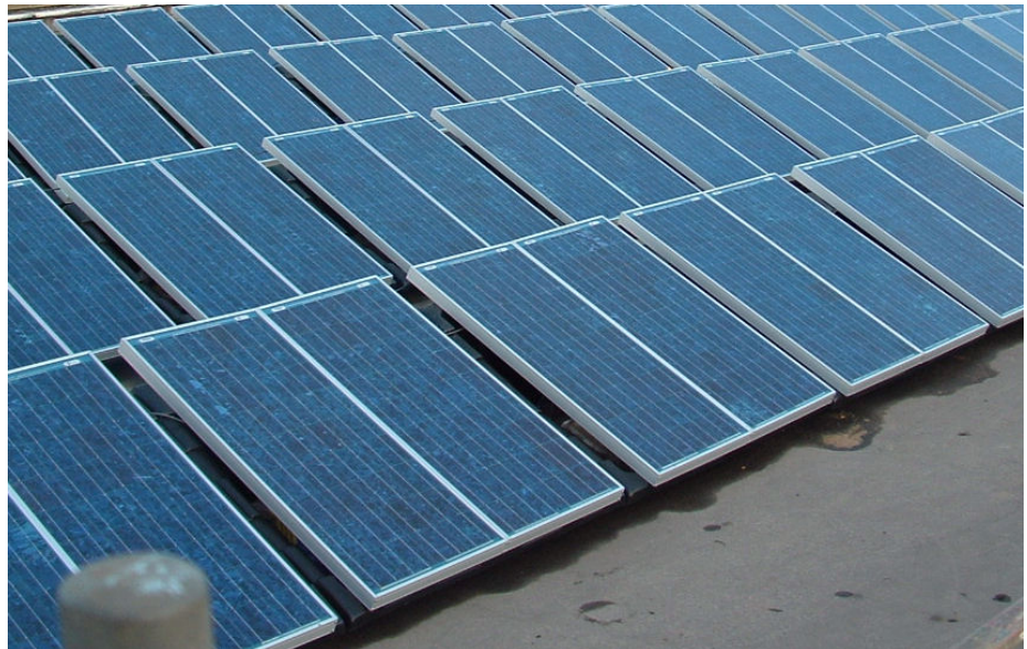
Solar Panels, Civic Centre 3, Kirklees
