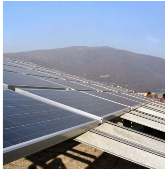
Solar Installation, Brescia, Italy
